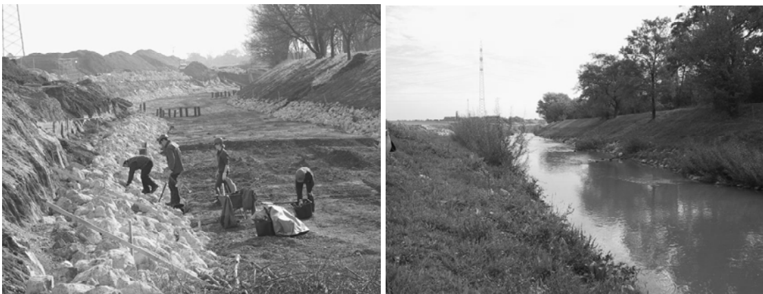
FIGURE 7: Construction of dormant cuttings and ecological groynes (left) and 2 years after (right)
