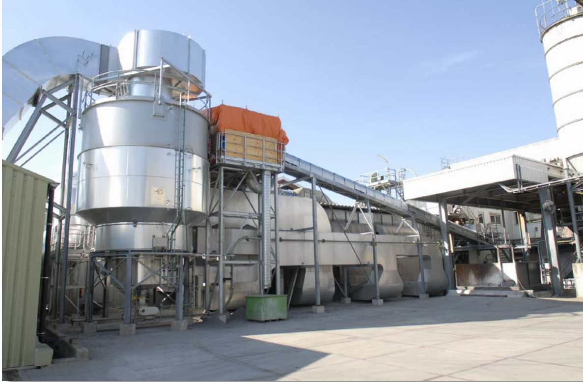
Figure 4: Compact Bed Reactor used as a paper sludge drier at a Sappi Mill in Holland
