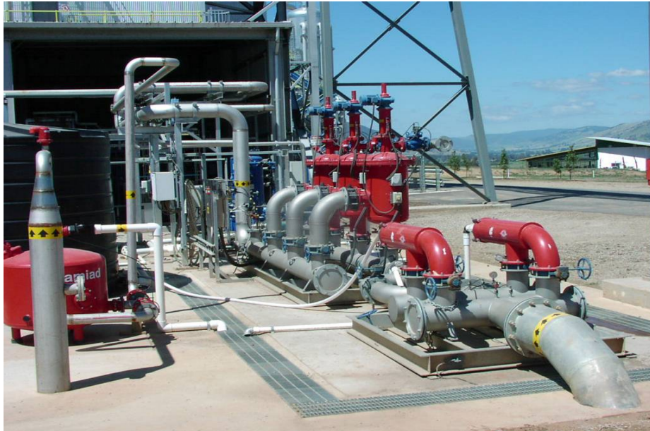
Figure 2: Filtration System at the Mill
